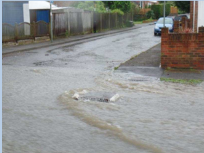
Figure 3 Surcharging manhole on Caterham Drive
